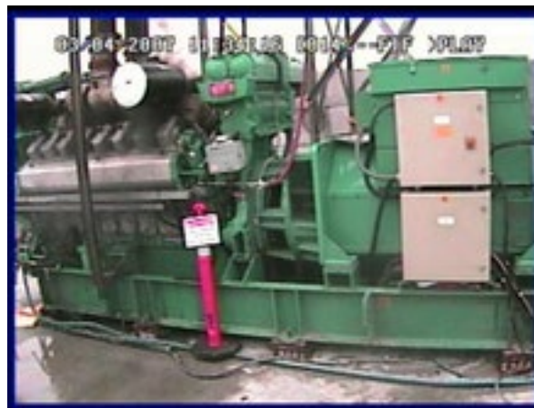
Figure 4 Aurora generator test
